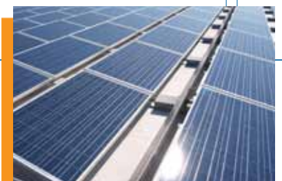
Photo courtesy of PanelClaw Inc.
